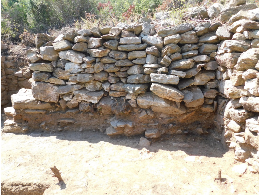
Figure 9. Poorly Built Southeast Wall
